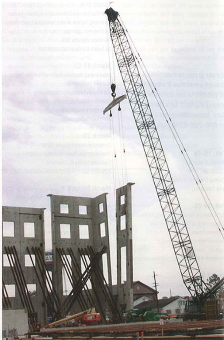
The tilt-up construction technique is expected to save about three months on the building schedule and up to 10 percent of costs for the Federal City building.
